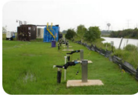
Groundwater Pumping Wells
