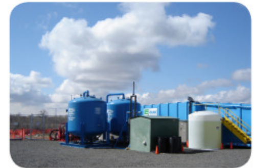
Outdoor Treatment Facility
